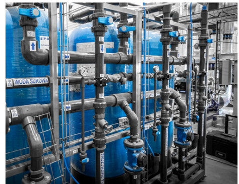
Water Supply & Sewage Systems
