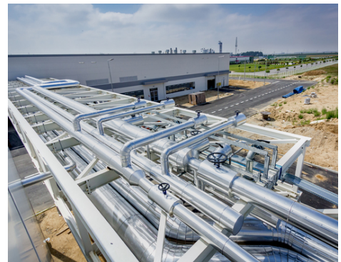
Technological & Industrial Installations
