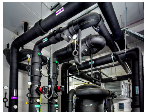
Heating & Cooling Installations
