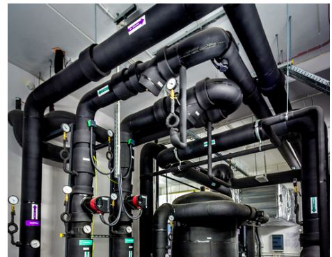
Heating & Cooling Installations
