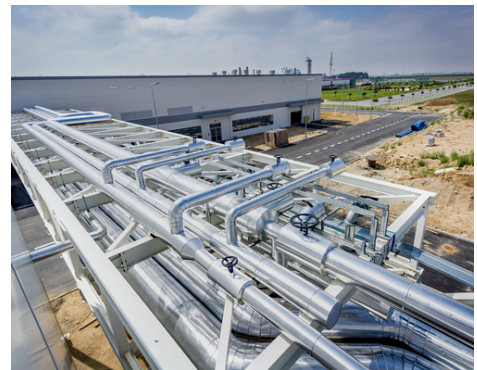
Technological & Industrial Installations
